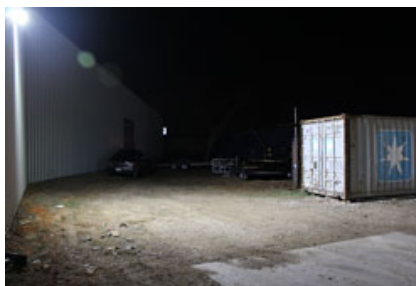
LEDWP-600E-OS mounted 15' high illuminating a 30' long by 50' wide parking area.
