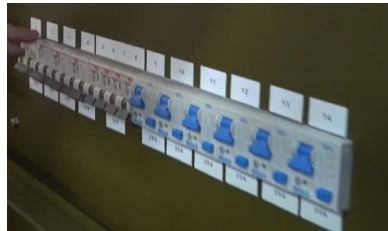
Low Voltage Breakers
