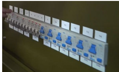
Low Voltage Breakers
